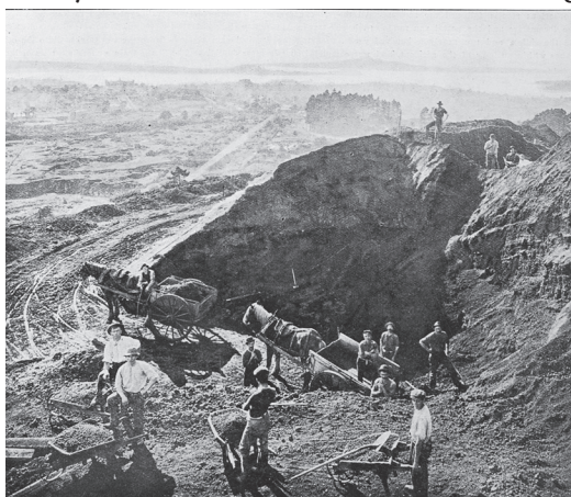
Horses and carts excavating for the new reservoir on Mount Eden in 1911
