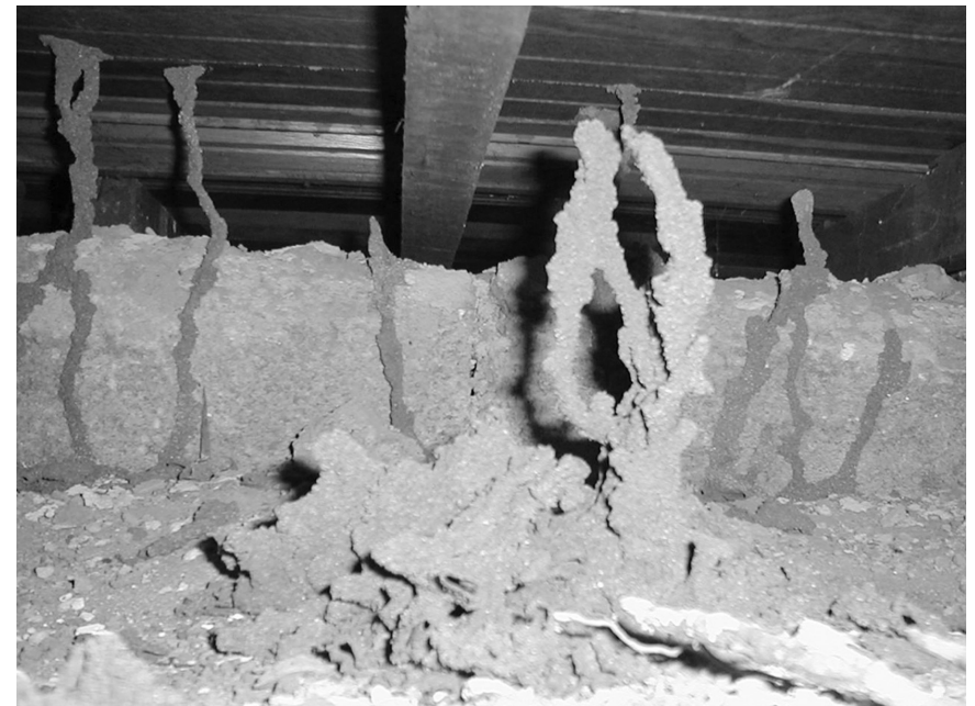
Elaborate 'leads' created by subterranean termites in their efforts to reach the timber
